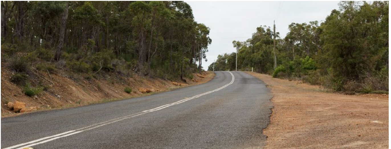
To significantly reduce serious crashes occurring on poor quality roads such as this, the Regional Road Safety Program if fully funded, would treat 17,000km of the State network with effective low-cost safety treatments including sealed shoulders and audible edge lines.
