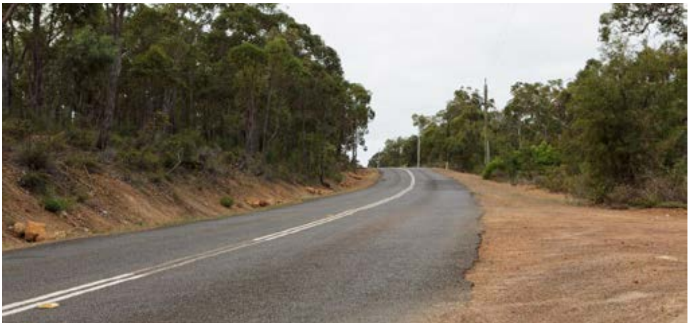
To significantly reduce serious crashes occurring on poor quality roads such as this, the Regional Road Safety Program if fully funded, would treat 17,000km of the State network with effective low-cost safety treatments including sealed shoulders and audible edge lines.
